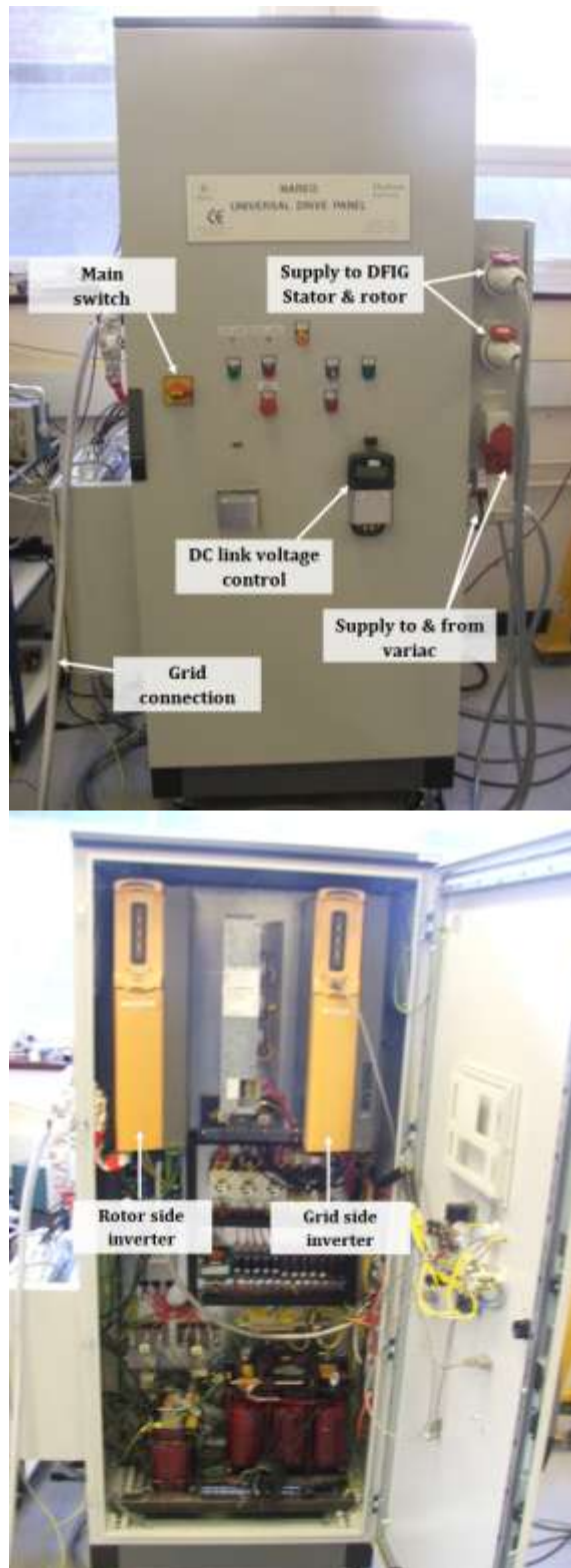
Fig. 3.4: Photographs of back-to-back converter cabinet
